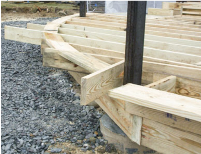
Figure 7. Where the joists would run nearly tangent to the edge of the deck, their supporting beam had to run as close to the deck's outer edge as possible.
