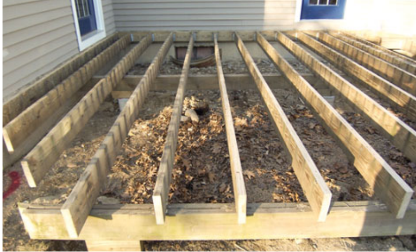
Figure 1. Still sound, the old joists needed only to have their tops planed flat in order to be reused.
