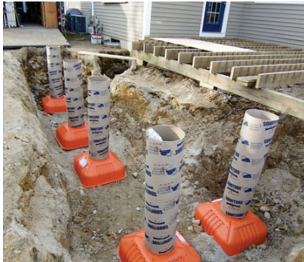
Figure 2. With an excavator on site for other work, setting the footings in a trench allowed accurate layout and minimal shovel work.
