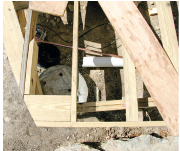
Figure 3. Careful planning meant that some footings could share loads from both the deck and the pergola.
